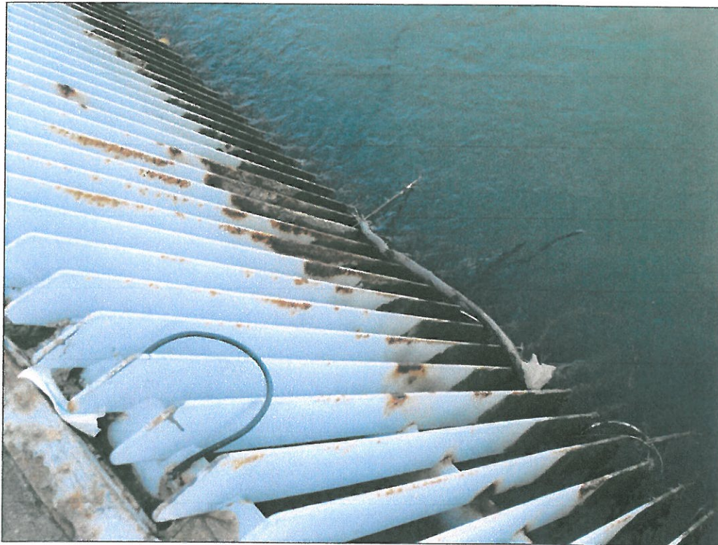
Upstream Trash Rack - Corrosion Example
